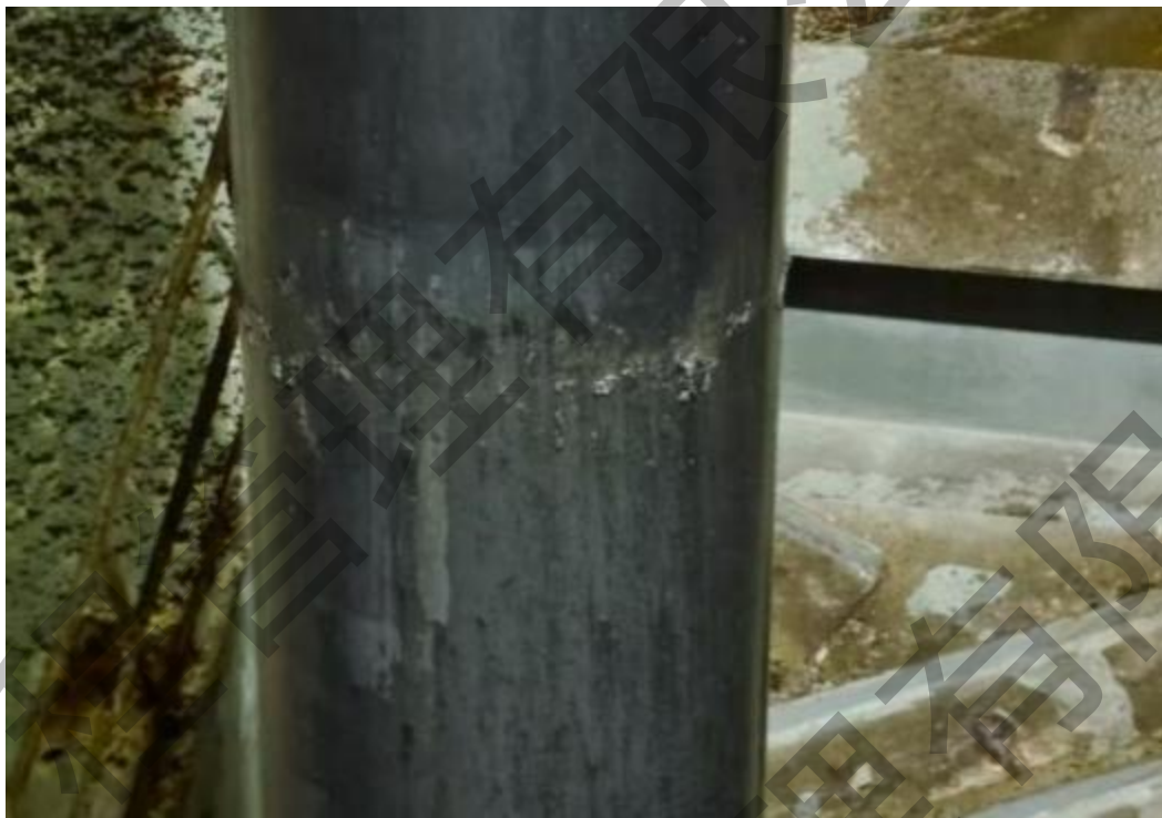
2#泄洪洞液压启闭机液压杆油渍、污渍
